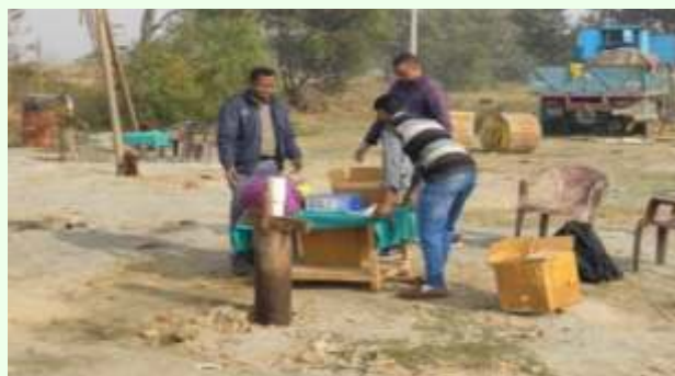
DWLR(with Telemetry) installed and tested at Banke bajar pump unit site, Gaya district, Bihar with CGWB officers and Engineers of Four ITS Pvt. Ltd.
