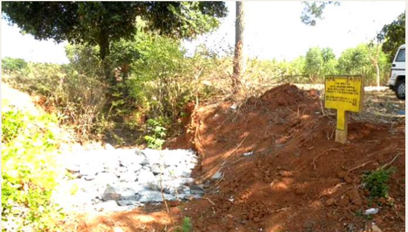
A boulder check constructed at the Kumudvathi river basin, supported by HAL
