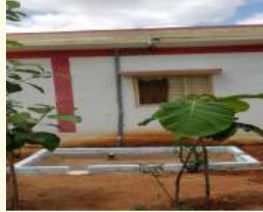
Rooftop Rain water harvesting structure at MPDO Office
