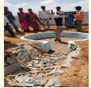
Borewell Recharge structure at Upper Primary School
