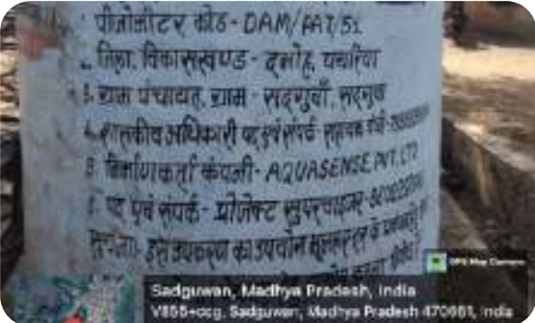
Piezometer installed in Madhya Pradesh
